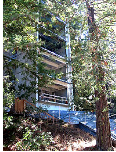
The three-building Humanities and Social Sciences Facility is scheduled for completion in fall 2006.
